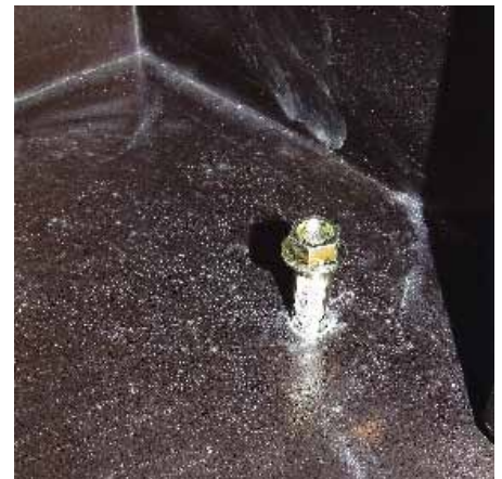
The dynabolts will need to be tapped into the hole with a hammer, but it is important to do this with the nut lightly screwed on to prevent losing the bolt down the hole.
